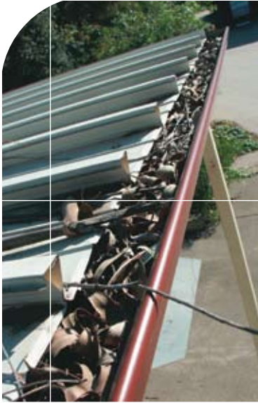
1) A typical suburban gutter clogged with leaf litter prior to cleaning.
