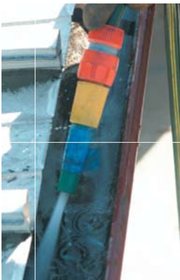
4) Rinse the gutter with water to soften and break up the dirt.
