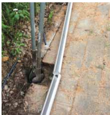
Lay the rails along the string line to determine positions of posts.
